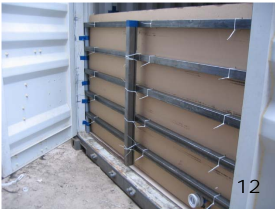
Center bar to stop metal bat from bending on pressure, Should be place in a way that the left door close on it. As In picture 14
